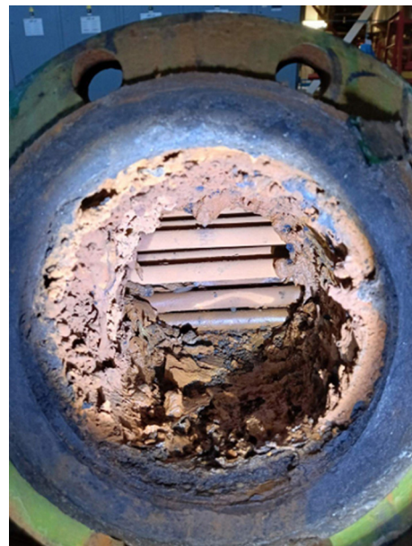
Fig. 6. Photograph of the external surfaces between the tube bundles of the heat exchanger before their cleaning
